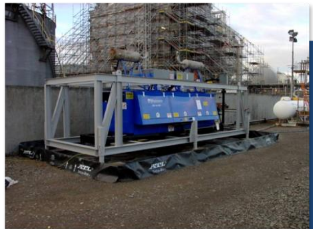
Skid unit in Grangemouth, Scotland
